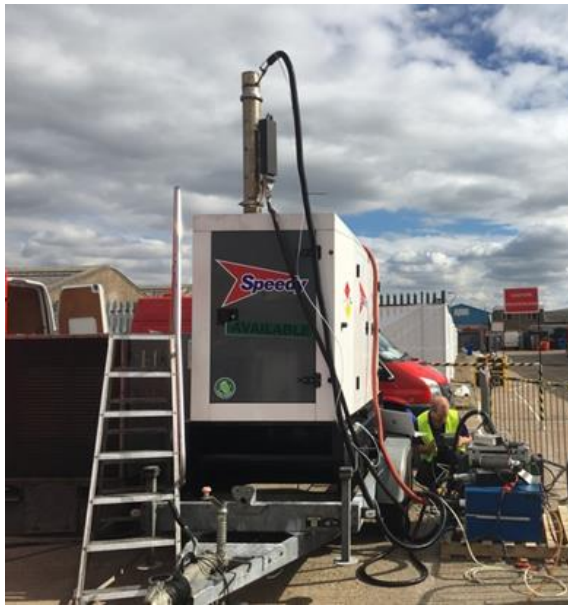
Figure 18 Generators being PEMS tested to characterise diesel emissions in the hire depot
